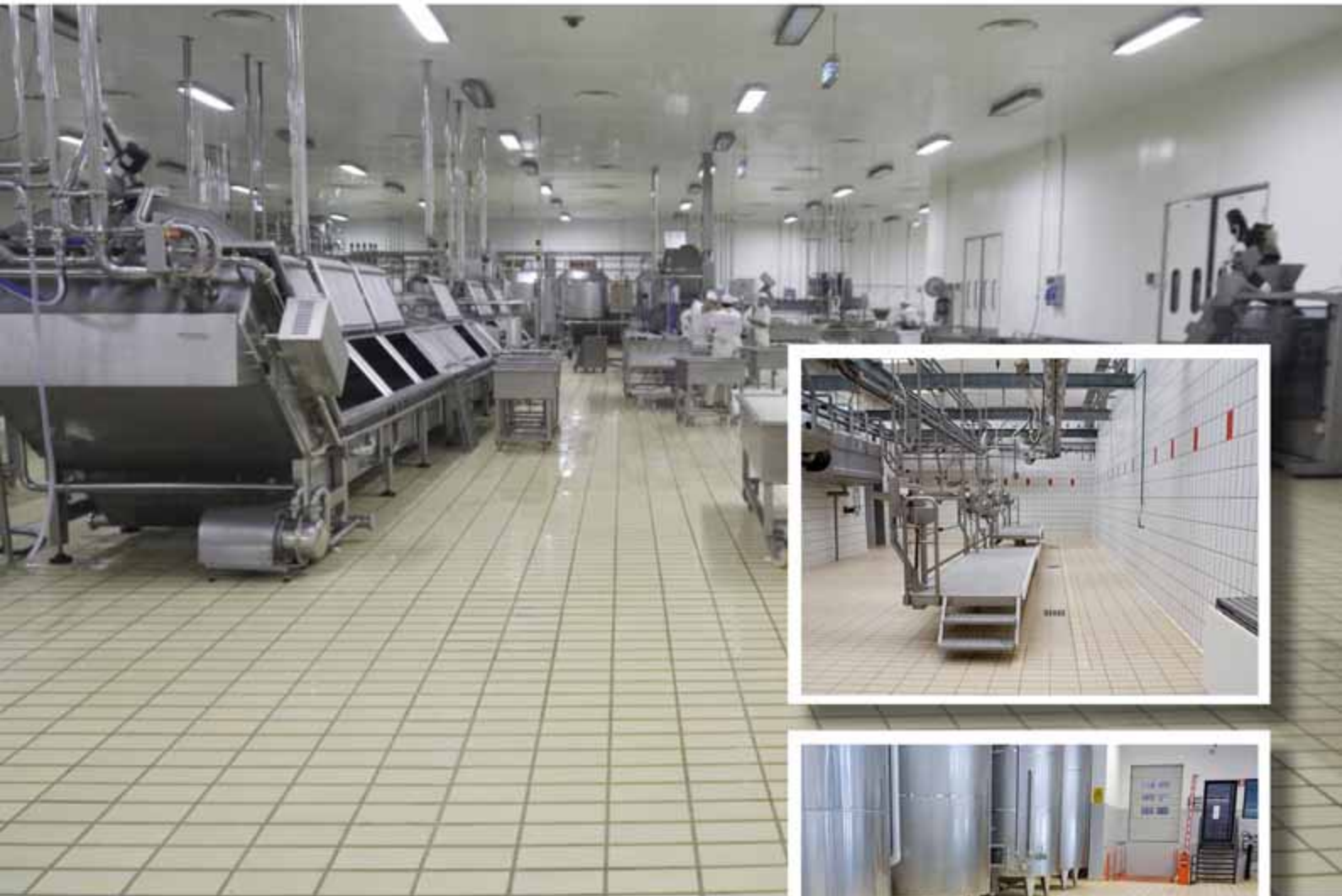
FOOD PROCESSING PLANT, UAE
